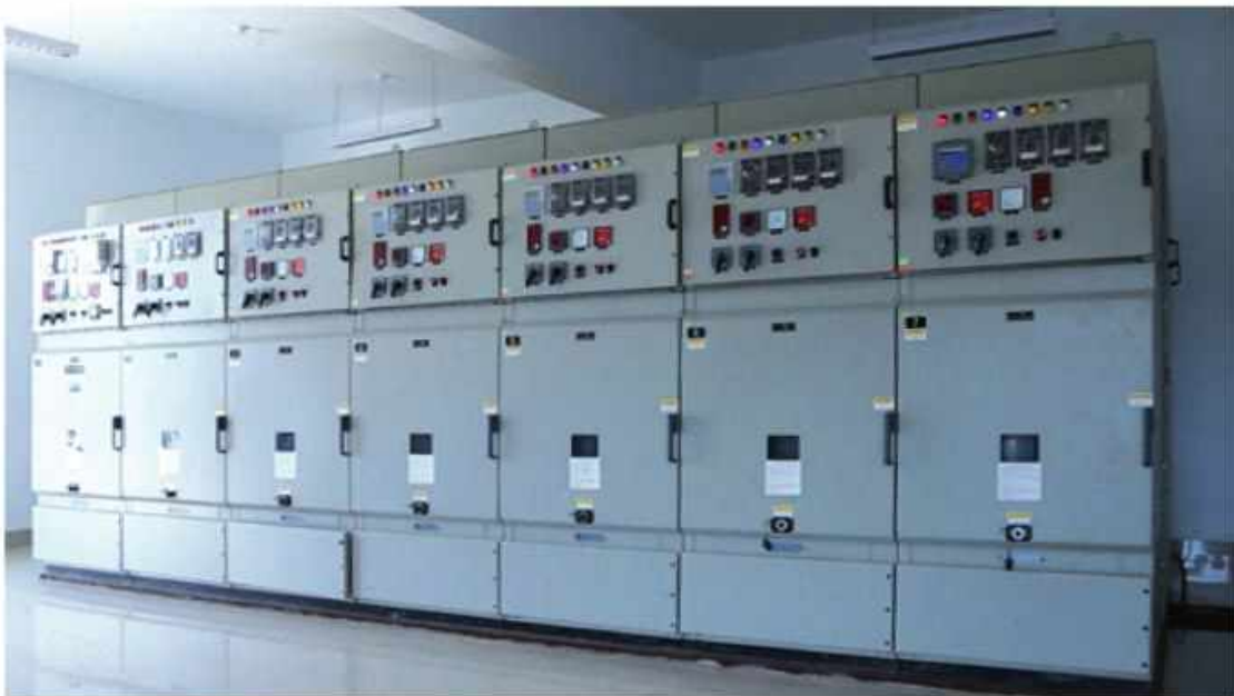
View: Control Room
