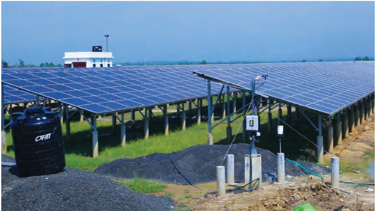
View: Solar Power Plant
