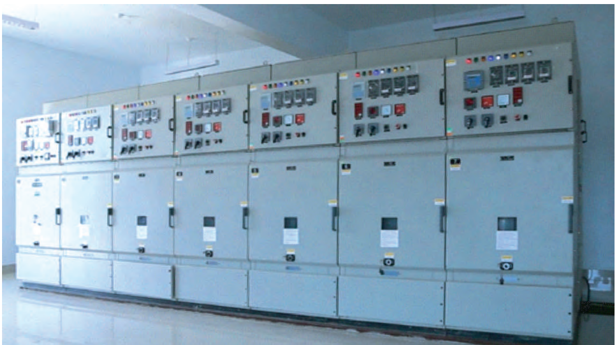
View: Control Room
