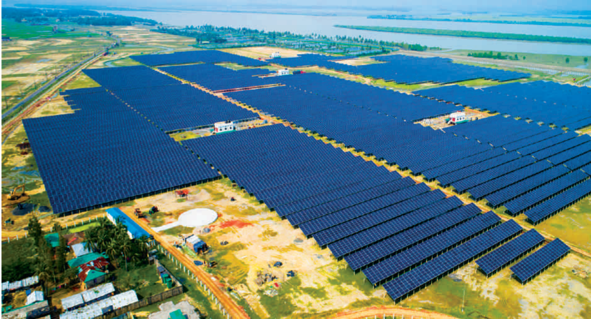
View: Solar Power Plant
